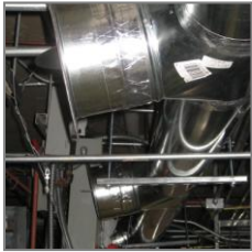
DIY waste-heat ductwork and fans
